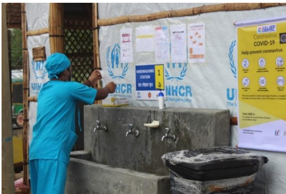
Handwashing facilities at UNHCR's Severe Acute Respiratory Infection Isolation and Treatment Centre in Ukiya. © UNHCR/Louise Donovan
