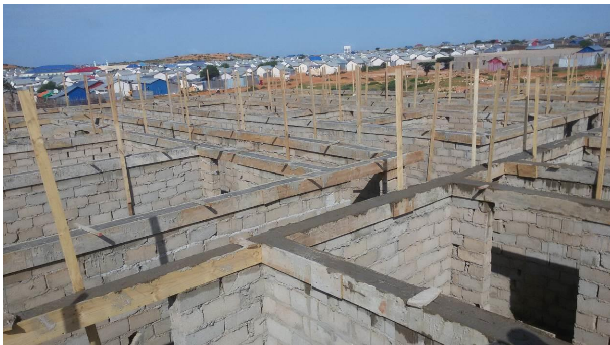
Construction of the Police Station at the new shelter settlement in Kismayo. © UNHCR/June 2018
