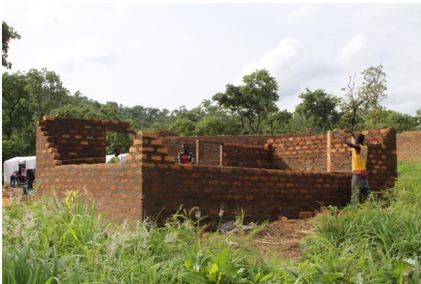
Cameroonian refugees building their shelter in Anyake settlement, Benue State © UNHCR / C. Cavalcanti
