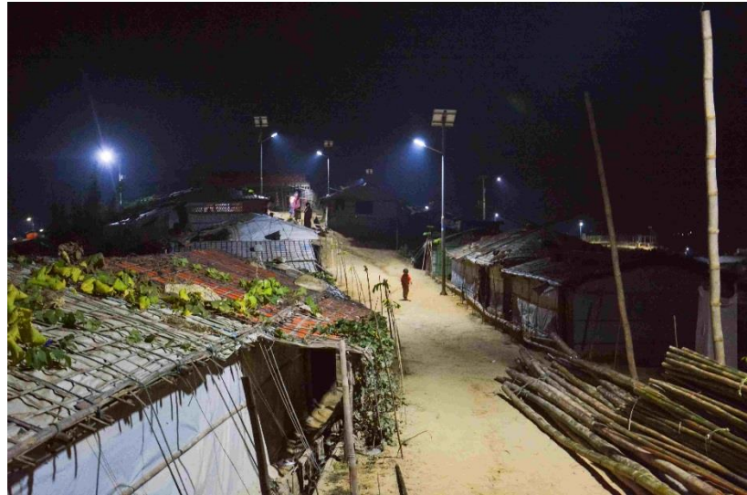
Street light illuminates public areas such as this road and prevents dark spots, therefore improving safety and community's sense of security. ©UNHCR/M. Edon
